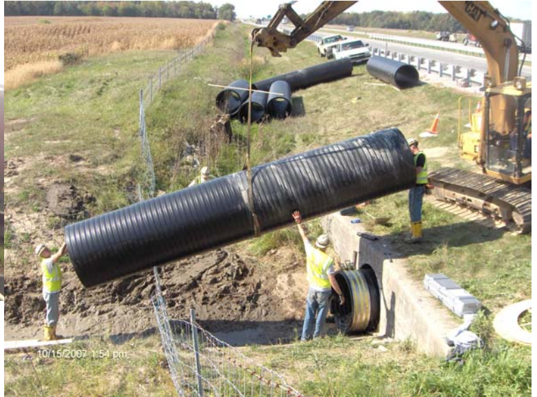
LOWERING A PIECE OF 42 inch HDPE PIPE FOR INSTALLATION INTO 54 inch CMP
